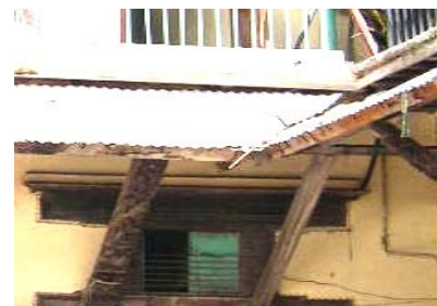
Plate 18: Missing strut replaced by ordinary
