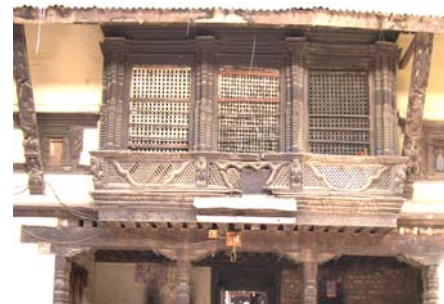
Plate 20: Existing ribbon window and Viman window from out and inside court respectively.
